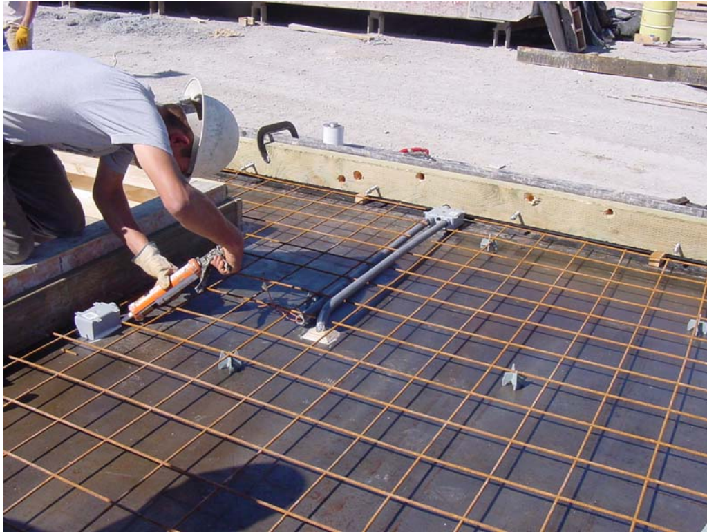
Figure 3. T-Mass wall assembly at the Precast yard. Thermocouples for the interior and exterior concrete of the T-Mass wall were placed in a PVC conduit which was cast into the concrete. An additional conduit was run to the interior of the wall for the installation of the wall heat flux sensor which will be run after the interior of the wall is finished. A junction box for the conduit was placed at the top of the wall to allow connections to the sensors.
