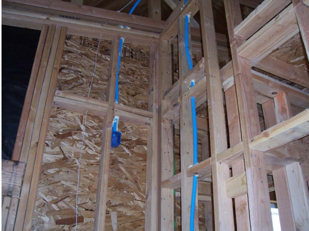
Figure 7. Blue non-metallic conduit (nmc) was run to the sensor locations in the walls of the baseline house. This aided in the pulling of the sensor wires and helps to protect the wires during construction. The conduit was run to the air conditioning attic access area. Penetrations through fire blocking and top plates were sealed with foam.
