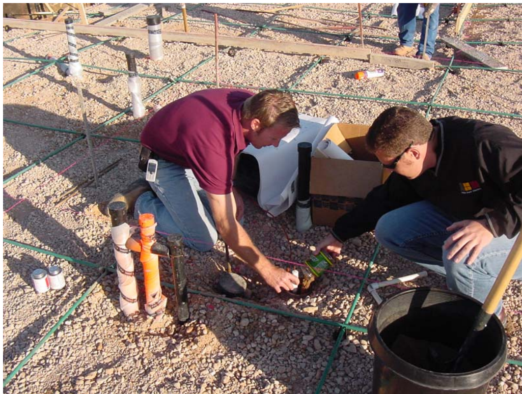
Figure 1. Placement of the floor sensors in the zero energy house before the concrete slab was poured. The thermocouples were mounted outside a small PVC pipe to maintain the depth below ground. This pipe was placed in a larger pipe which kept the hole from backfilling. After the sensors were placed, the hole was filled with sand, compacted, and the larger pipe was removed.
