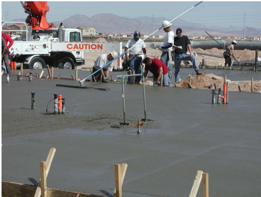
Figure 2. Concrete slab pour for the baseline and zero energy house. The slab and underground thermocouple leads can be seen in the center of the photo. The connections will be made in a j-box located in an interior wall.
