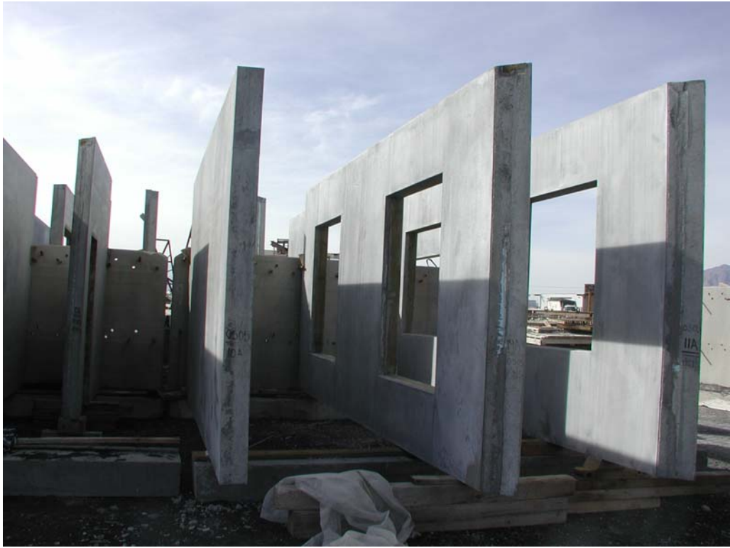
Figure 5. After the T-Mass walls were poured there were stood in the Precast yard to allow the concrete time to cure.
