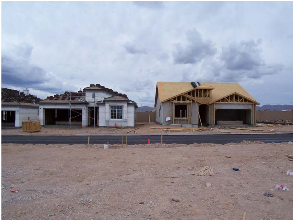
Figure 8. Front exterior view of the baseline house (left) and Zero Energy House (right) during construction.
