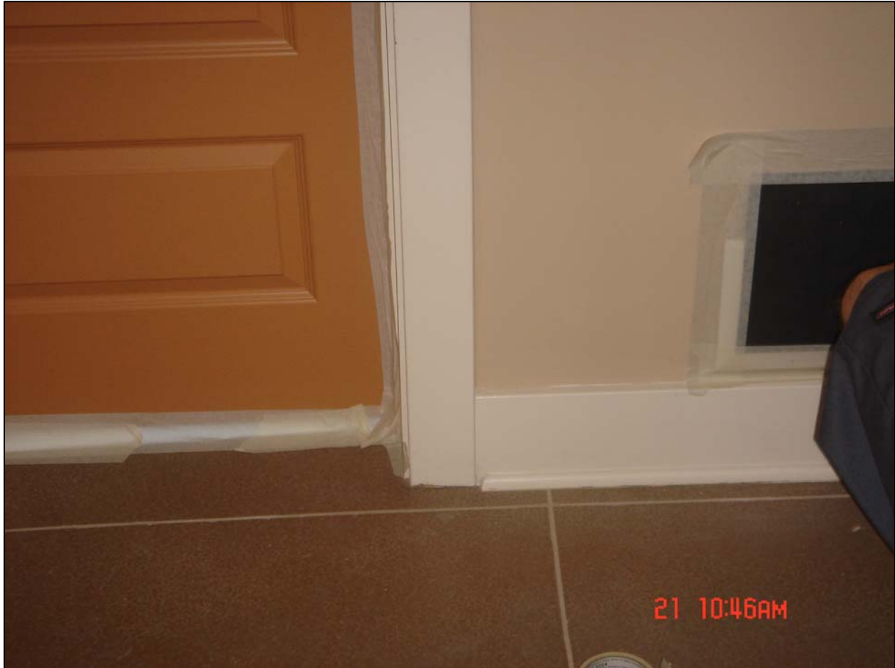
Figure 9: Floor to Wall Infiltration Gap
