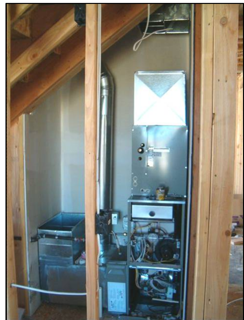
Figure 8 Air handlers located inside the heated space for the Condact (left) and New Traditions homes.
