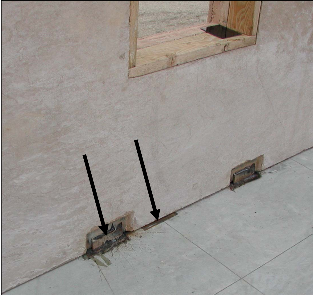
Figure 16: Incorrect Weld Plate Placement
