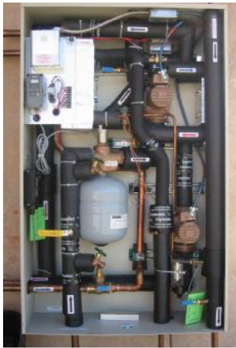
Figure 7: Hydronics Module for the Wagon House
